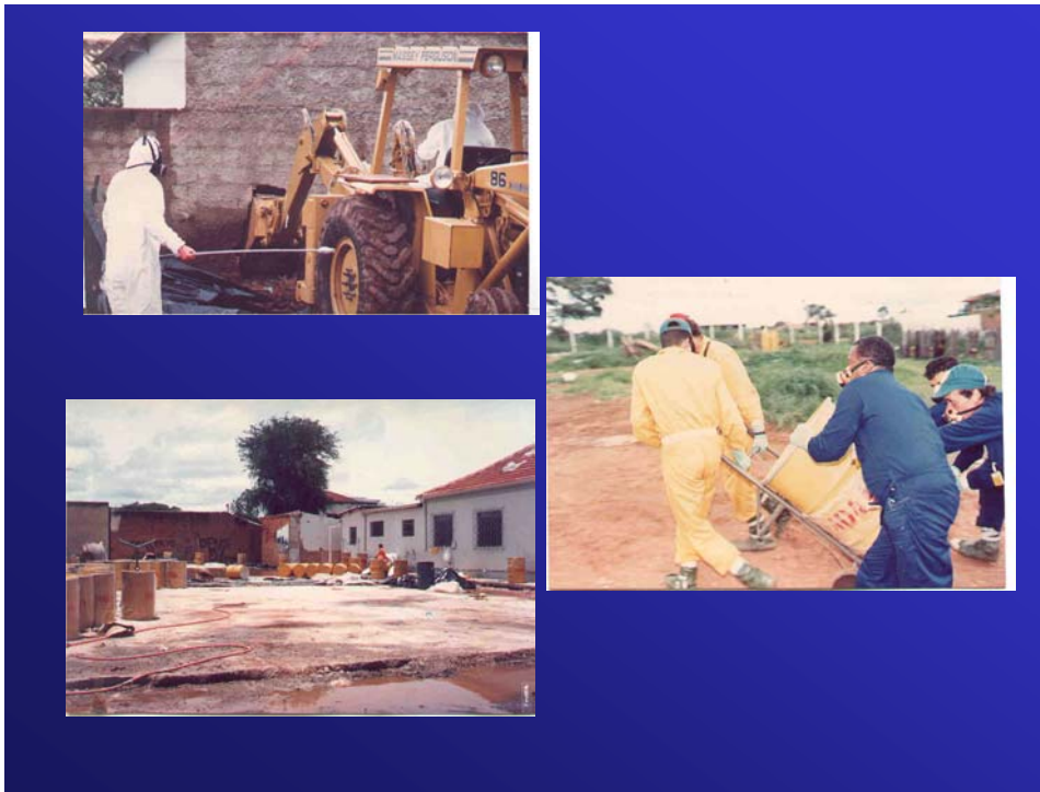
Photos of the scrap yard, demolition of a building and carting of contaminated soil.
